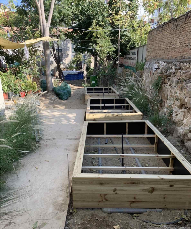
The farmers module with the water system installation © Gardens of the future Photo Archive
